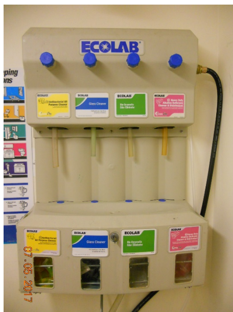
Figure 7 - Ecolab Chemical Premix Station
